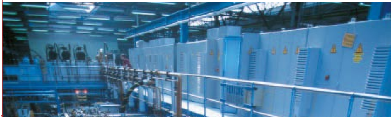
Overview of the Hayes-Lemmerz wheel rim line consisting of reeling, welding and profiling units.
